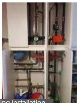
An existing installation
