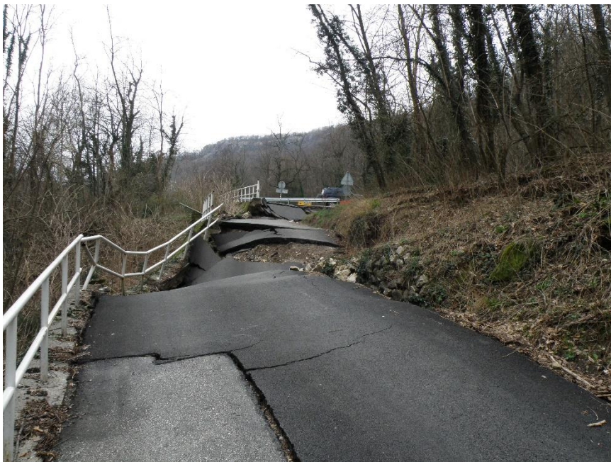
Figure 1. Road damages caused by landslide
